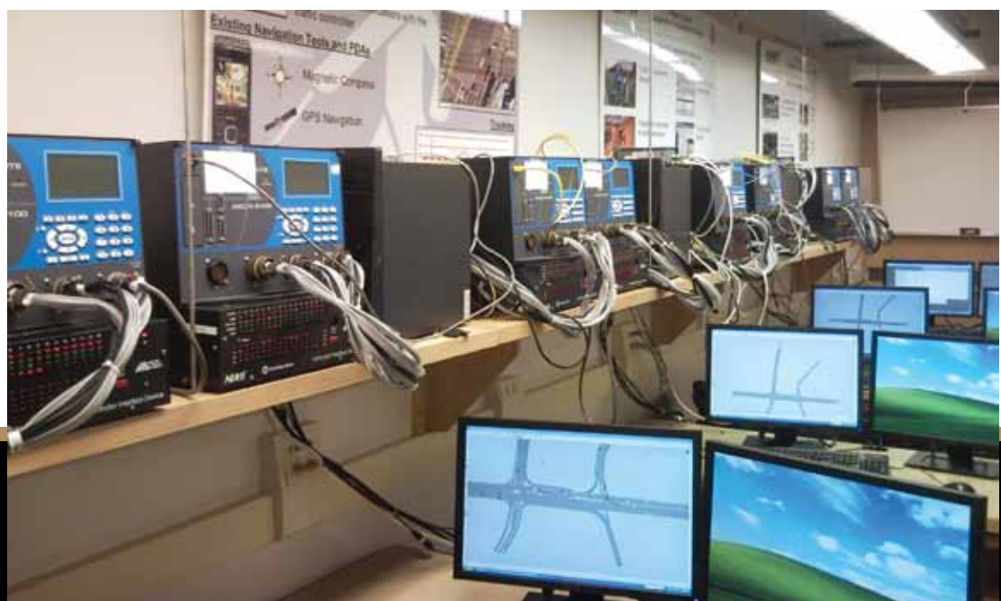
Traffic controller network in the NIATT computer lab.
