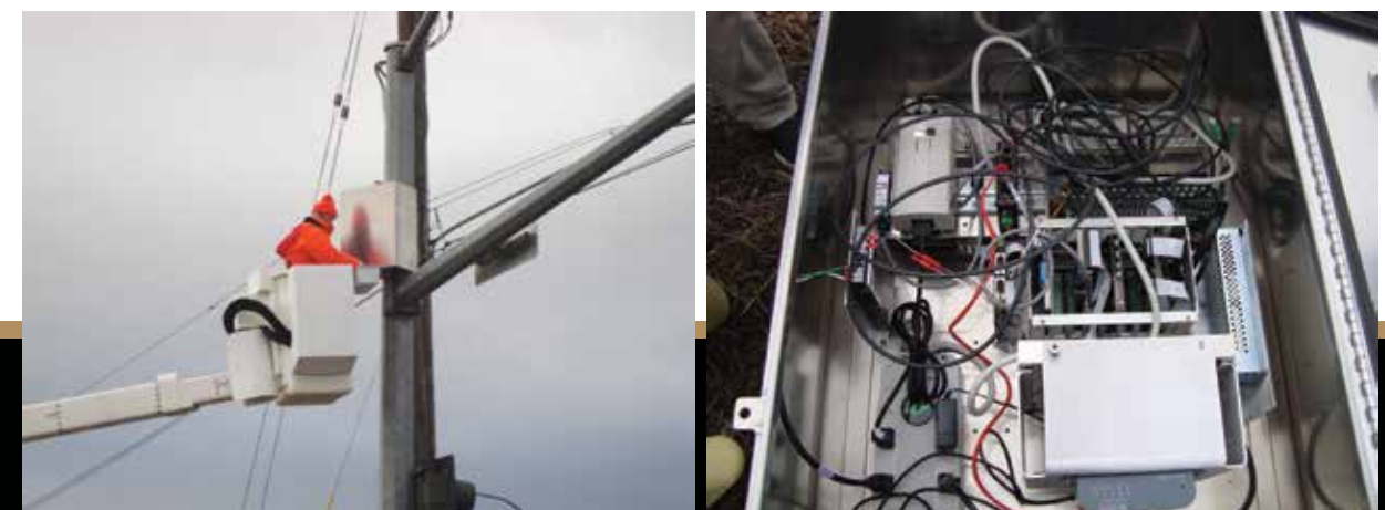
Left: Field installation of the local weather station. Right: Components of the local weather station.
