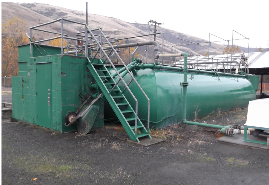
Figure 21. City of Juliaetta centralized wastewater treatment plant, 2017.
