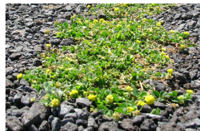
Figure 1. Black medic invading cracks in blacktop pavement. Courtesy of Forest and Kim Starr, Starr Environmental, Bugwood.org.
