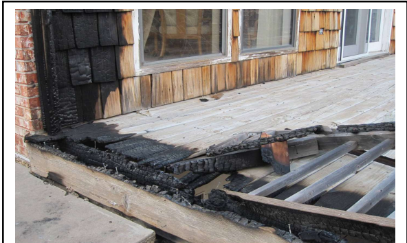
Combustible decks that aren't treated with fire-resistant paint or chemicals are more likely to catch fire.
