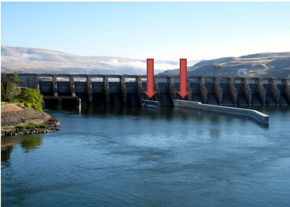
Figure 1. Photograph of spill walls at bays 6-7 (left) and 8-9 (right) at The Dalles Dam in 2010.
