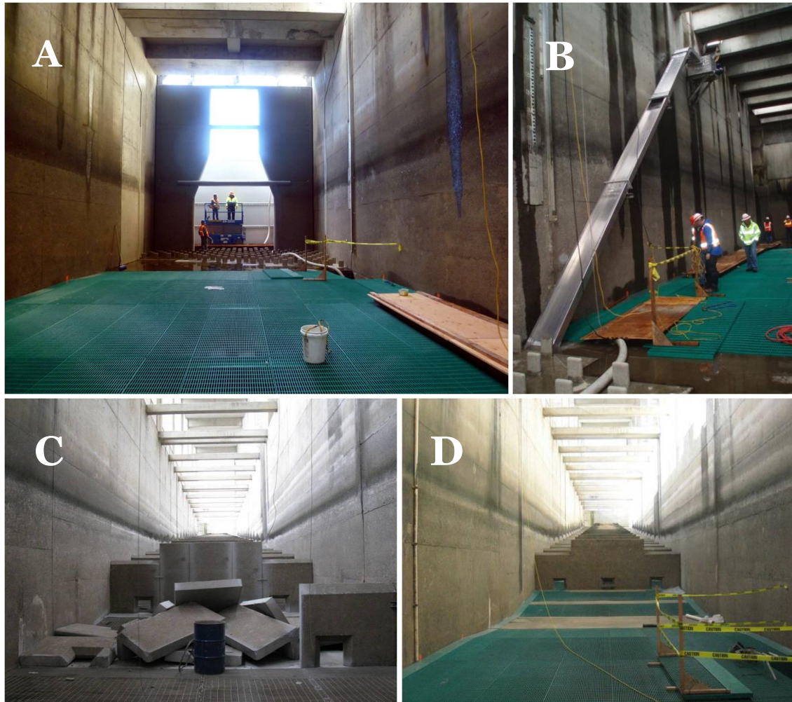
Figure 2. Modifications to the John Day Dam north fishway entrance area; camera is facing upstream in all photos except A. From left to right, clockwise: A) downstream variable-width entrance weir, bollard field, and closed entrance slot (new concrete on left wall); B) lamprey passage structure (with bollard field in foreground); C) removal of concrete weirs; and D) completed fishway with concrete weirs removed.
