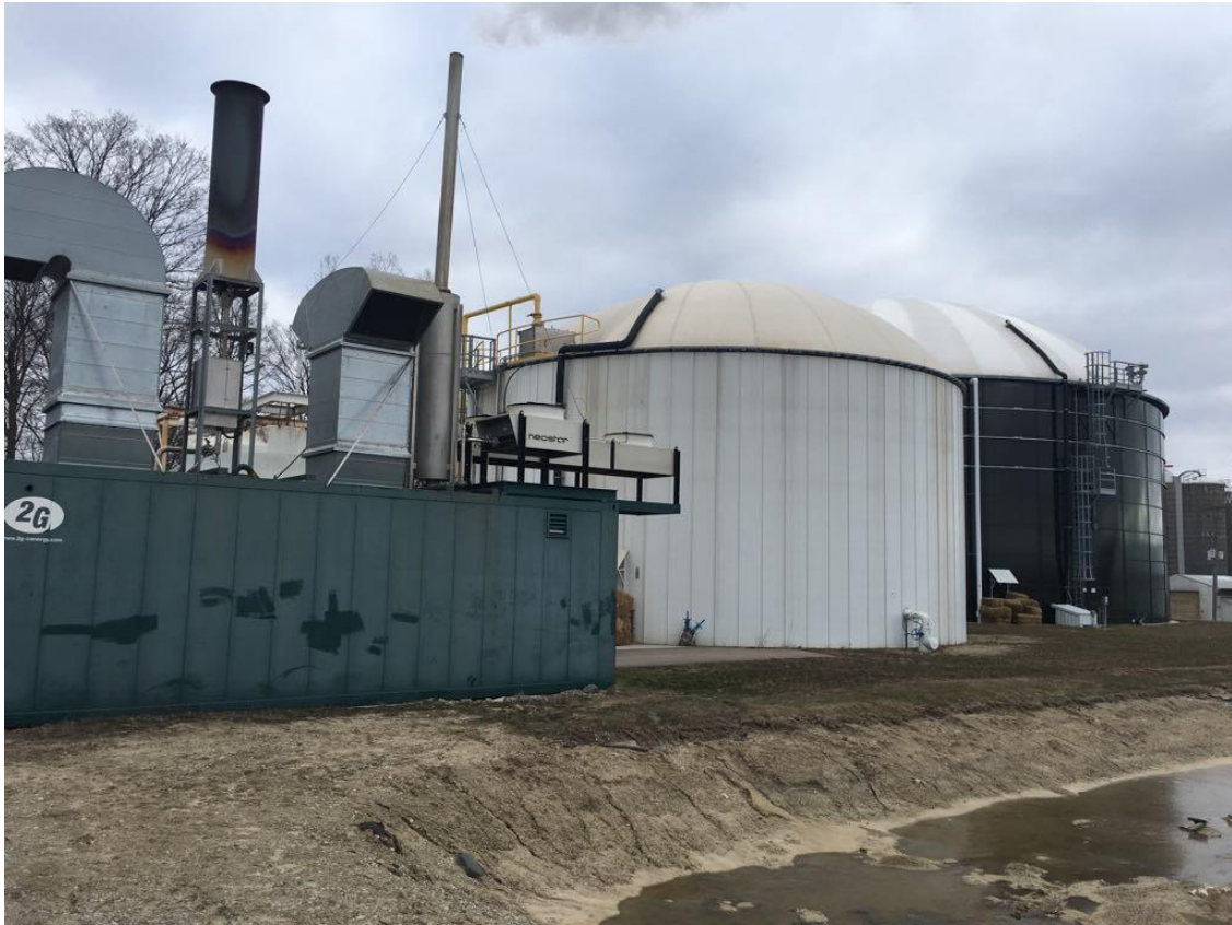
Figure 8: MSU biogas facility
